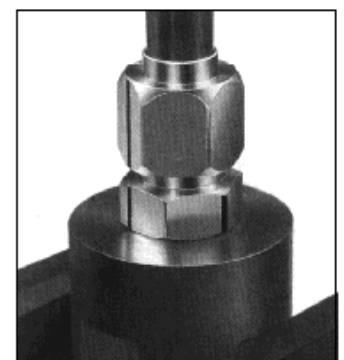
Fully tightened positioned with displaced mark example shows a nut at 1 1/2 flats from finger tight.
